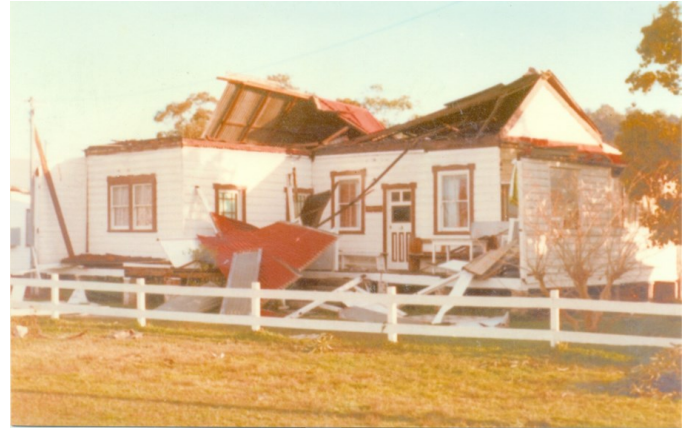
Roof damage along Sorrento Road
